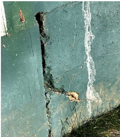
Figure 7 – Crack in Front Steps
