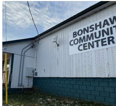
Figure 2 – Wood Siding at End of Life
