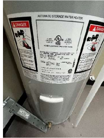
Figure 18 – Hot Water Tank
