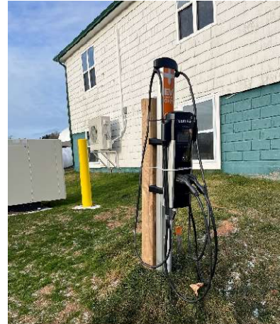
Figure 22 – Charging Station for Electrical Vehicles
