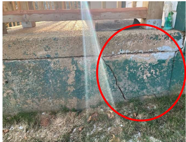
Figure 8 – Crack in Front Steps
