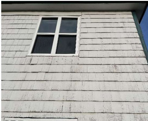
Figure 1 – Paint Peeled on Siding
