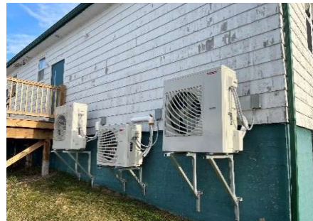
Figure 4 – Paint Peeled on Siding
