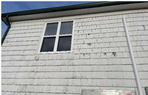
Figure 3 – Paint Peeled on siding
