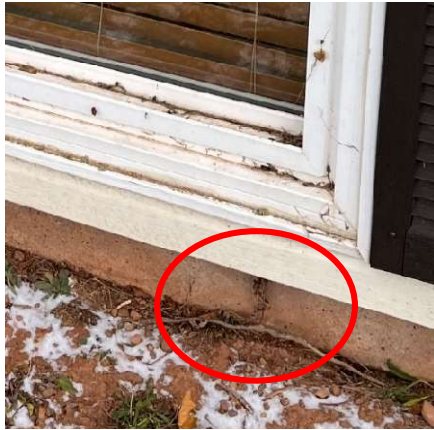
Figure 7 – Cracked Window Frame
