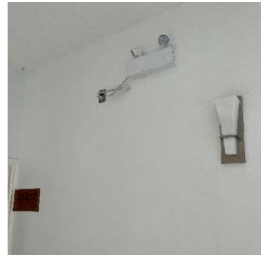
Figure 25 - Emergency Light and Wall Sconce
