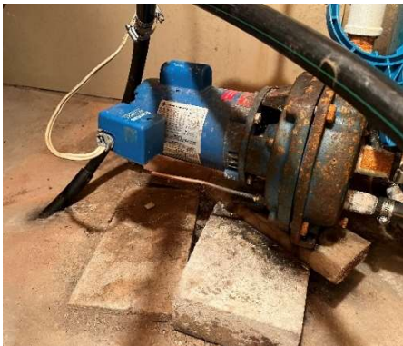
Figure 12 – Pump Near End of Life
