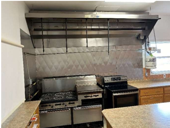
Figure 28 - Kitchen Range and Fire Suppression
