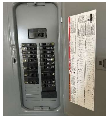
Figure 21 – Electrical Box (100 Amp) in New Building Addition
