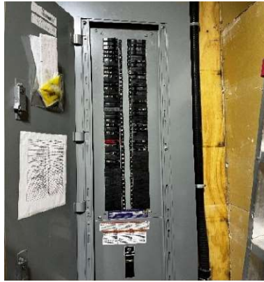
Figure 18 – Main Electrical Panel (225 Amps)
