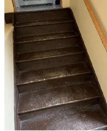
Figure 36 - Wooden Stairs Require Paint
