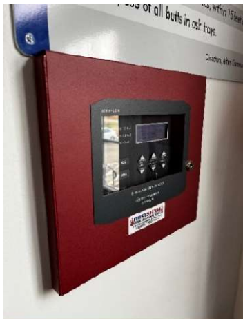
Figure 37 - Central Alarm Panel
