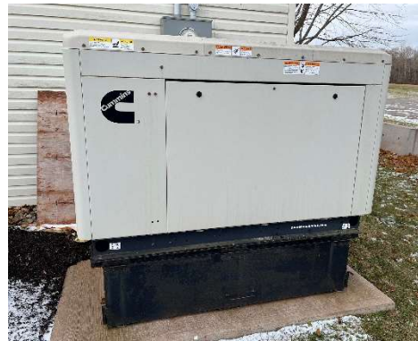
Figure 23 – Cummins Propane Generator
