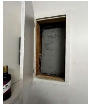
Figure 19 - Junction Box (Kitchen)
