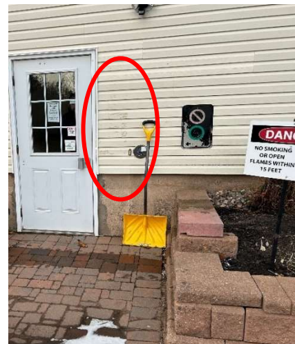
Figure 4 – Dirt Accumulation and Wear
