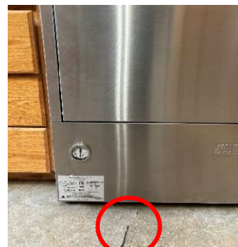
Figure 34 - Kitchen Floor Damaged
