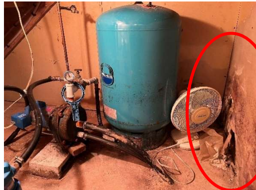
Figure 13 – Pump Area - Mould Removal and Repair Required
