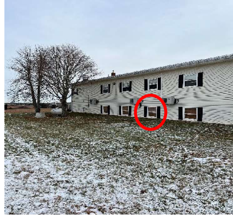
Figure 8 – Location of Foundation Crack
