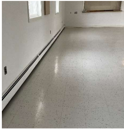
Figure 35 - Upstairs Multipurpose Room Floor - Light Wear Only
