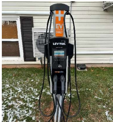
Figure 22 - Charging Station for Electrical Vehicles.
