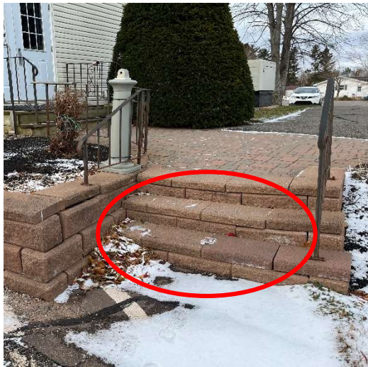
Figure 10 – Main Entrance - Steps Settling
