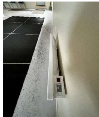
Figure 32 - Significant Wear - Side Entrance Hall
