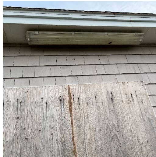
Figure 12 - Exterior Fluorescent Lights
