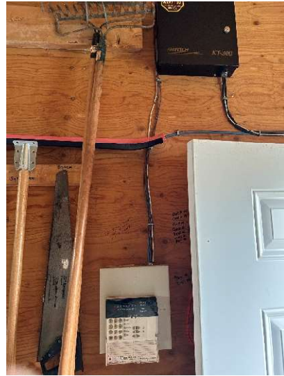
Figure 18 - Mechanical system alarm.
