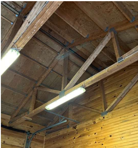
Figure 11 – Fluorescent Ceiling Lights
