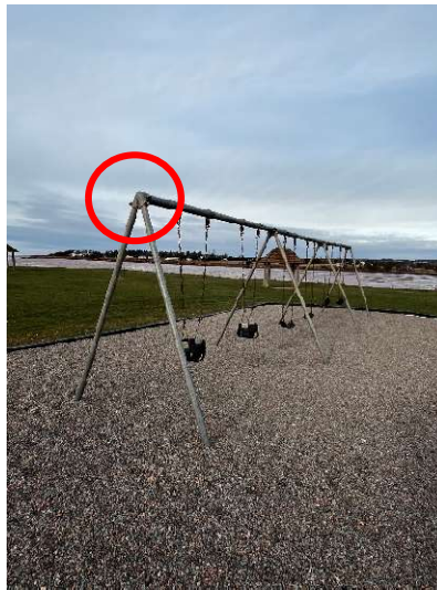
Figure 10 – Rust Forming on Swing Set
